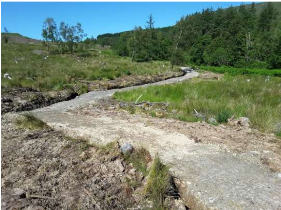
As dug trail – completed just weeks ago – one contractor with one 5T excavator using borrow pits to provide all formation and surfacing (holes used to bury cleared soil, stumps and harvesting residues)
