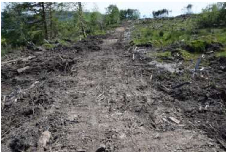
A future internal network of forest trails (for walkers but also compact tractor/trailer forest management) is planned – following roughed out forwarder tracks. Possible use of recycled membranes and as-dug materials to make all ability spec.
