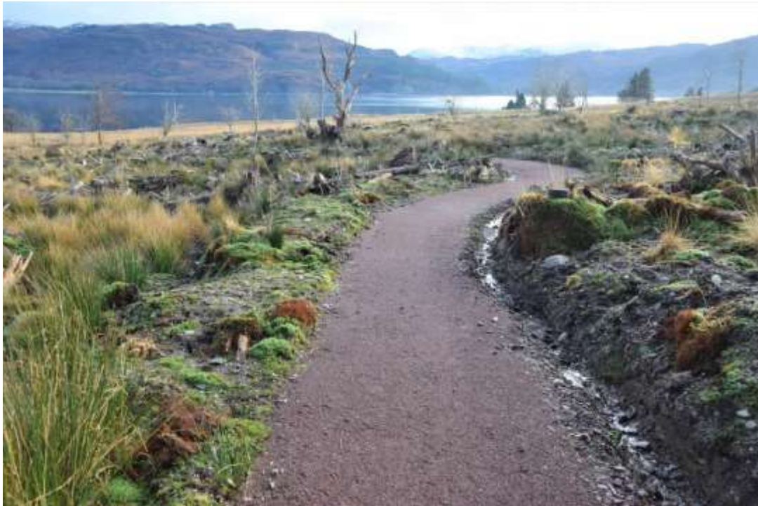
All-abilities trail – a circular pram/wheelchair accessible path around old Kirkton village ruins and new wildlife pond – 2 contractors using 5T digger, 1T dumper and whacker plate and all imported stone for formation and surfacing
