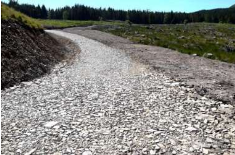
New timber haulage road to Cat1A forest road specification - constructed using one operator with 16T excavator, 8T dumper and roller – all formation and surfacing materials won on site from adjacent 'rotten rock' quarry cutting
