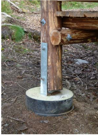
Fig 2. Detail of the galvanised steel plates supporting the uprights and reducing the opportunity for water to contact the end grain (photo: Sunart Oakwoods Initiative)
