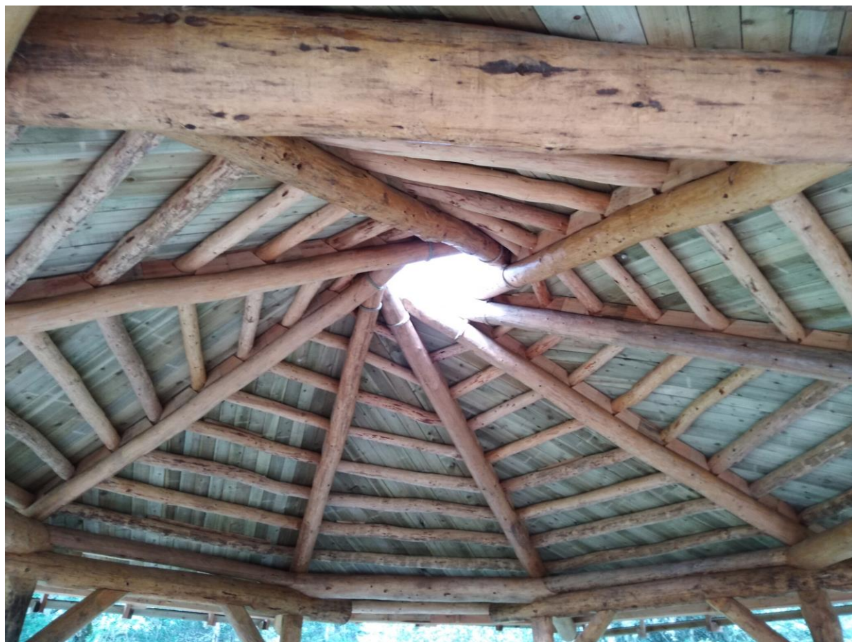
The reciprocating log roof of Evanton Wood Community Company's new woodland shelter.
